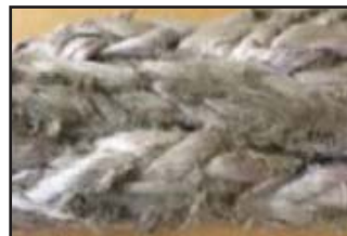
Excessive External Abrasion
